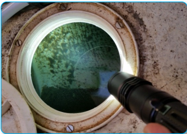
Water tank with biofilm
