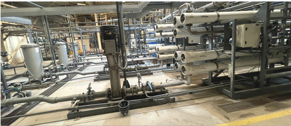
Industrial water treatment plant with pre-filters (left) and membrane filters (right)
