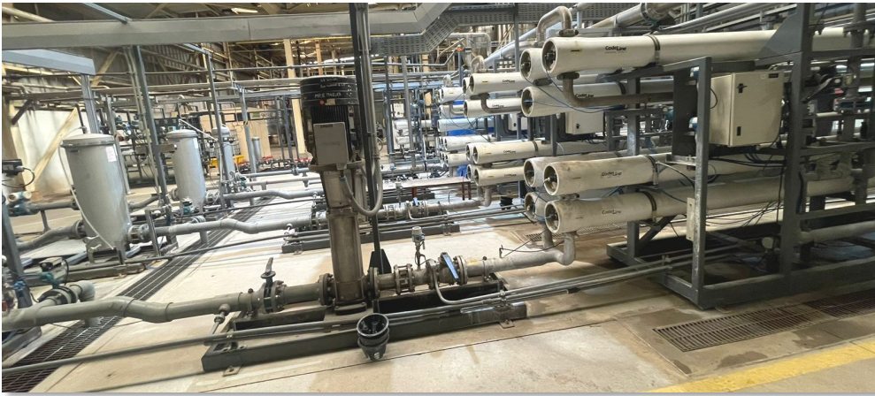
Industrial water treatment plant with pre-filters (left) and membrane filters (right)
