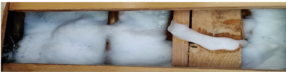
Biocidal foam made of SFS and Sanosil S015 in floating screed after water damage with subsequent mould infestation.
