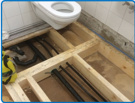
Water damage with faecal water, toilet, intermediate floor flooded
