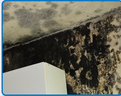
Water damage with mould development, cellar room after flooding
