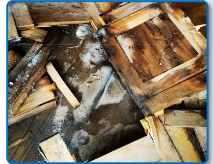
Water damage with mould development in intermediate floor (wood)
