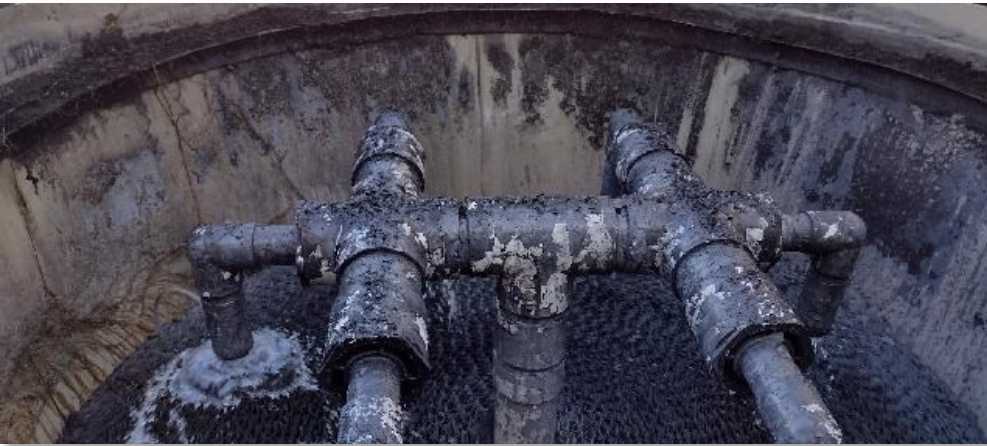
Evaporative cooling system with strong lime and dirt crusts
