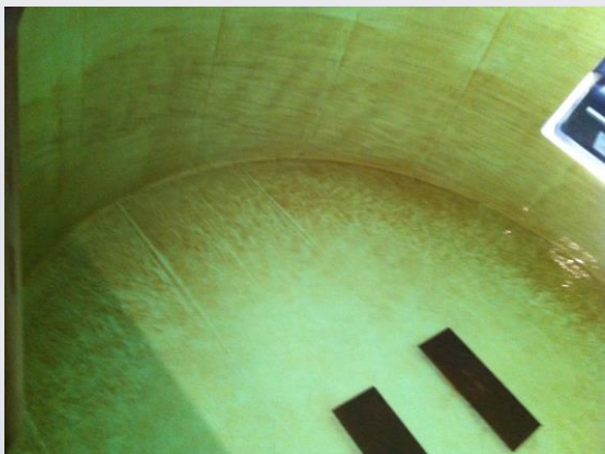
Drinking water chamber with deposits
